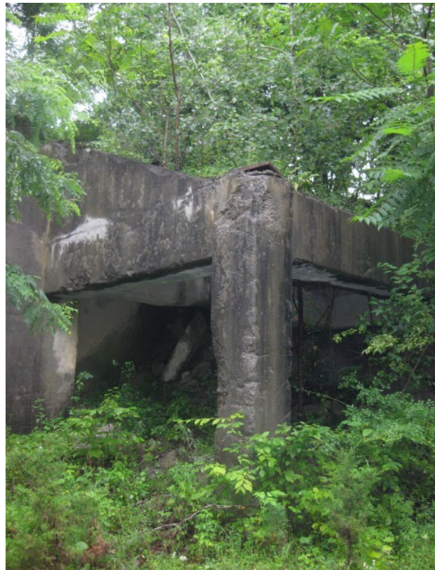
Figure 27. Photo of concrete foundation (c. 1937) of crusher used to reduce cement stone for use at Universal Atlas' cement plant in Greenport, New York.
